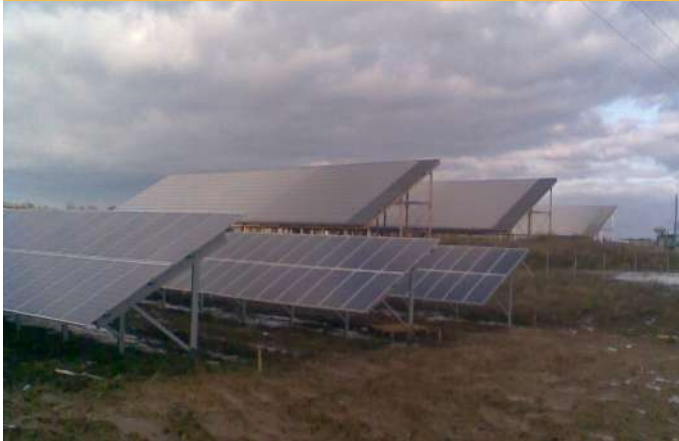
7,2 MWp, Germany, Kodersdorf 2012 Client: Reninger
