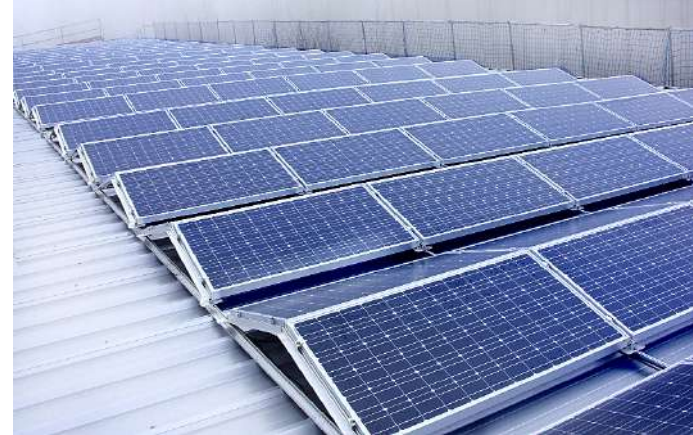
960 kWp, Germany, Kaufbeuren, 2014 Client: Dachsolar
