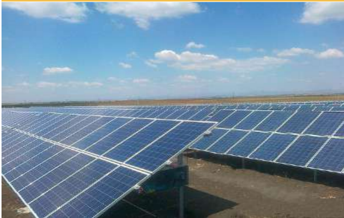
2,7 MWp, Greece, Agios Prodomos 2014 Client: Union Solar
