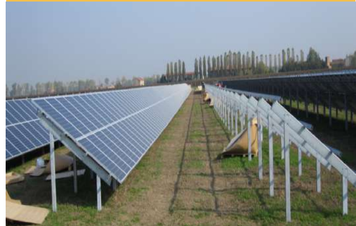
3,8 MWp, Italy, Collabria, 2012 Client: Municipality
