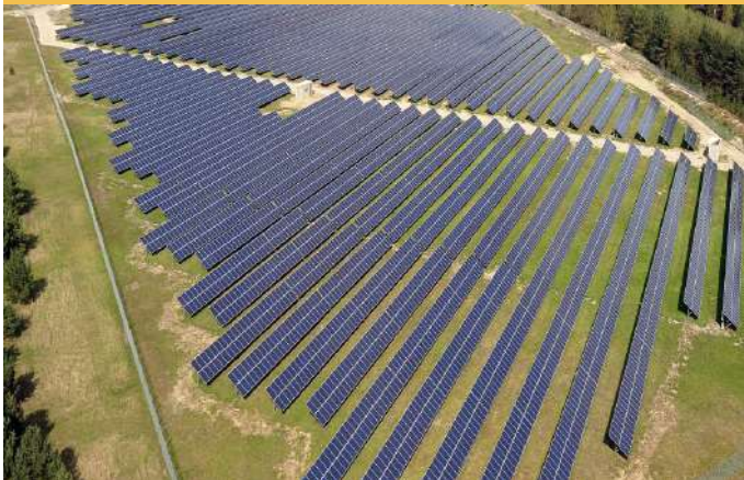
10 MWp, Germany, Pritzen, 2016 Client: Ahtos-Gruppe
