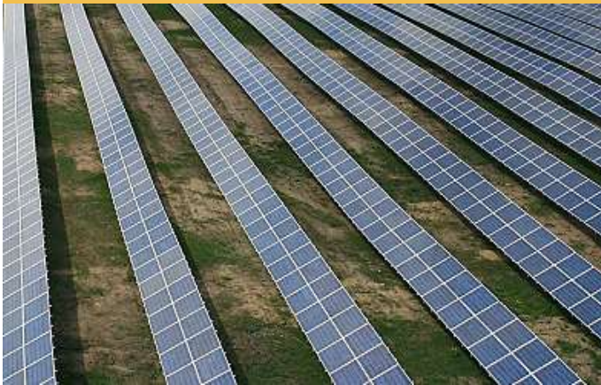
9 MWp – Bulgaria, Sliven, 2011 Client: Technomash
