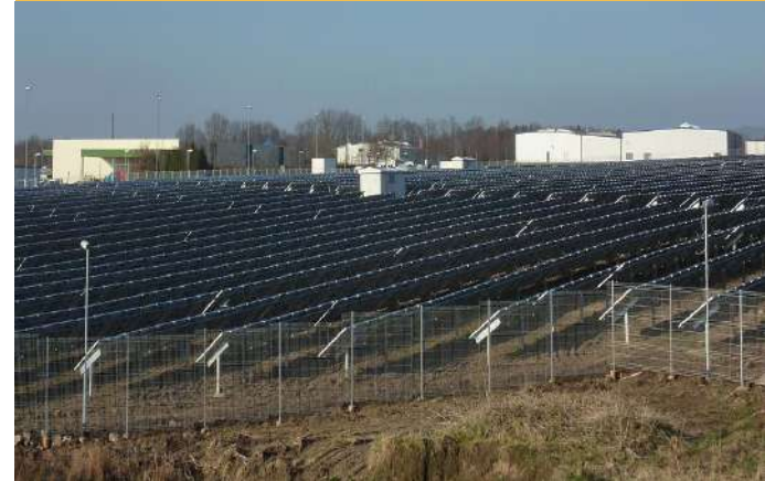
3,7 MWp, Germany, Kittlitz, 2013 Client: TK Gruppe
